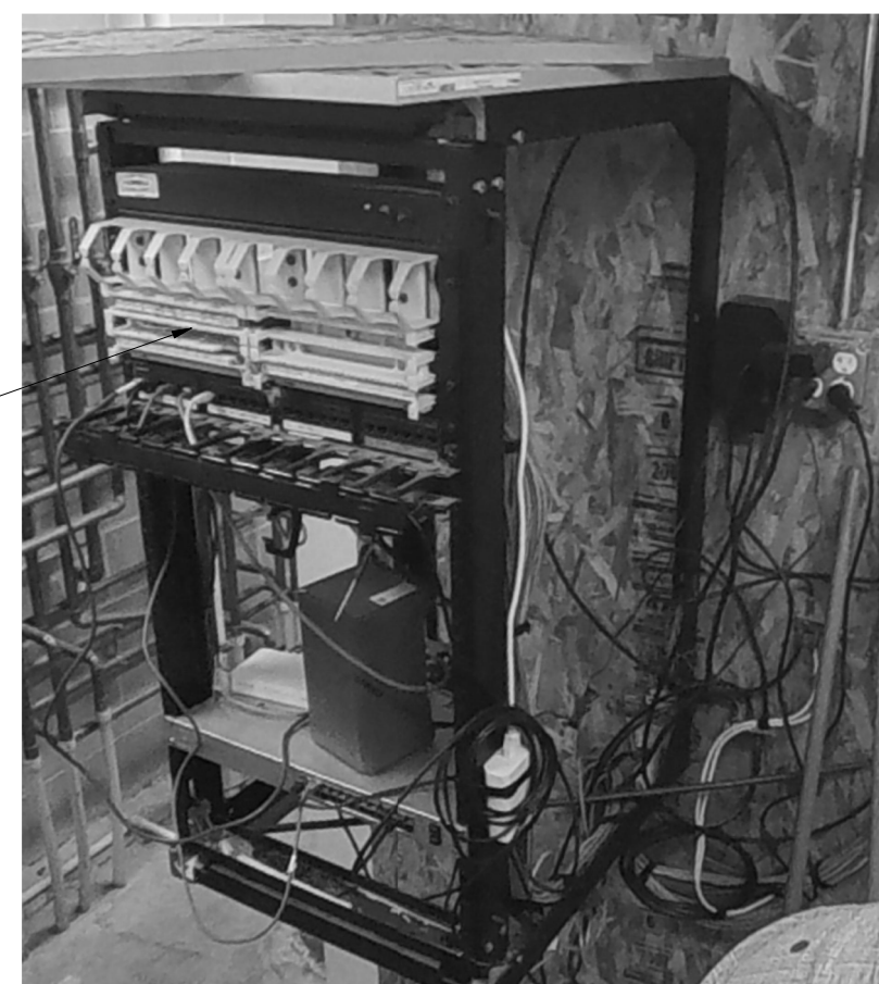
FIRESTATION - EXISTING DATA RACK
