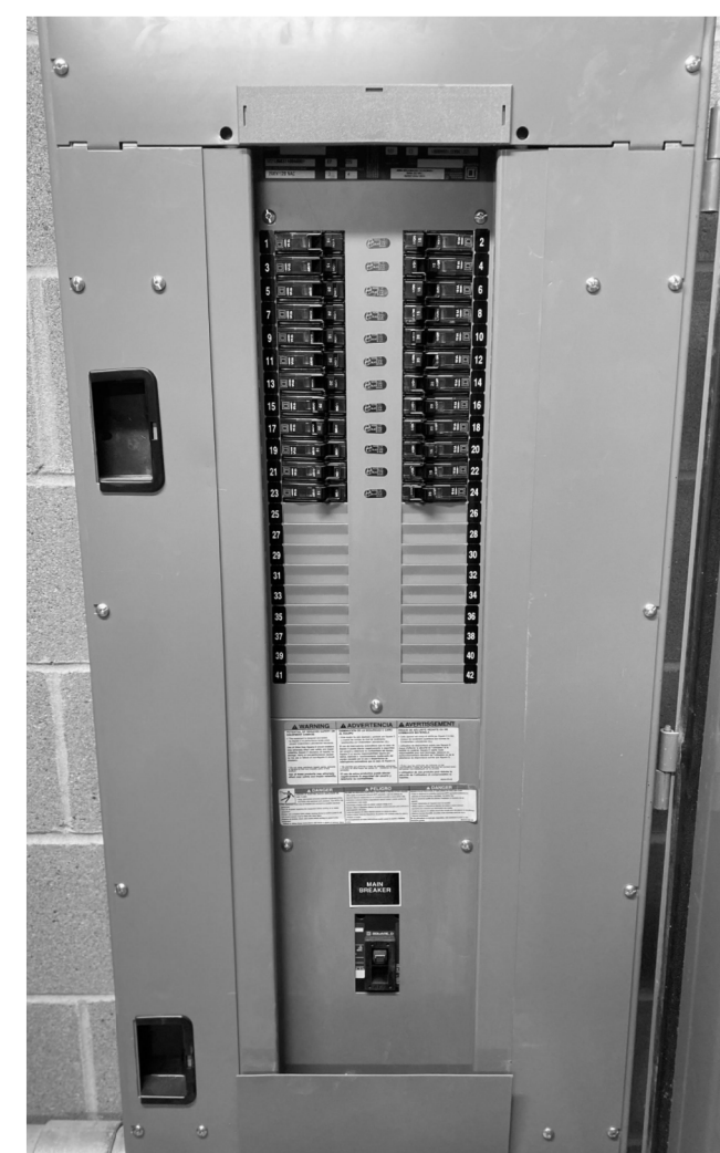
SQUARE-D PANEL. PROVIDE (3) NEW 20A/1P BREAKER IN SPARE SLOT. PROVIDE THREE SETS 3/4" CONDUIT AND 2-#12 & 1-#12 GND TO ACCESS CONTROL PANEL DATA CABINET AND MONITORING PANELS. LABEL NEW CIRCUITS ON PANEL SCHEDULE
