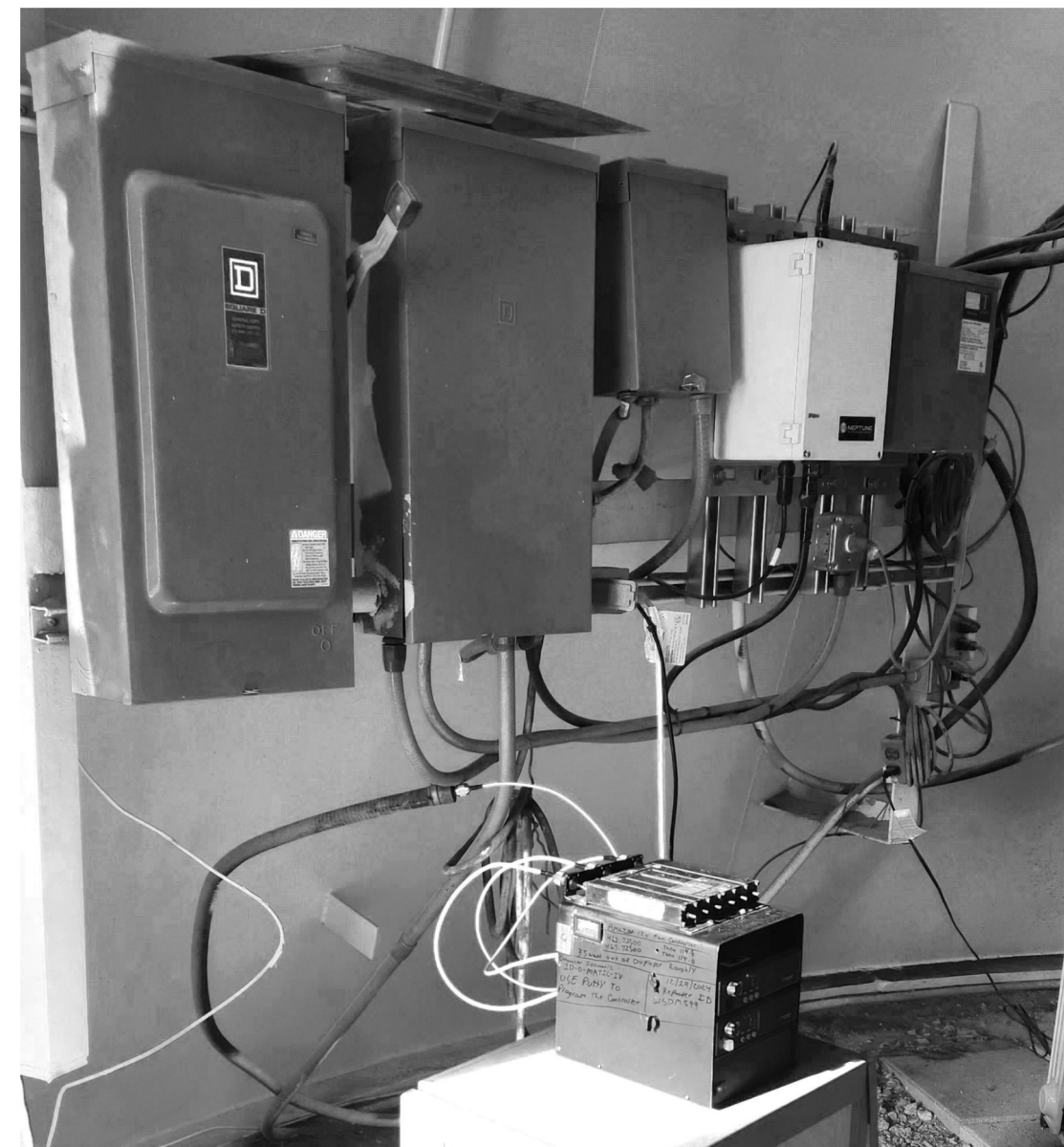
SQUARE-D PANEL. PROVIDE NEW 20A/1P BREAKER IN SPARE SLOT. LABEL NEW CIRCUIT ON PANEL SCHEDULE
