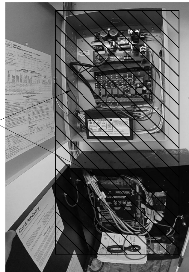
FIRESTATION - EXISTING ACCESS CONTROL PANEL
